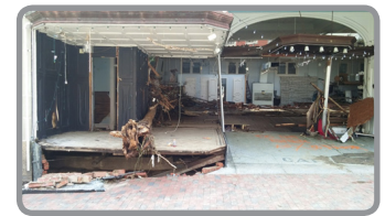
Damage to a store in Ellicott City, MD from flash flooding on July 30. Credit: National Weather Service (LWX).
