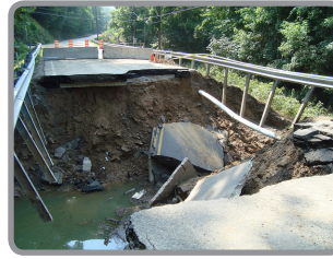
Damage from flash flooding in southern West Virginia on June 23. Credit: WV Dept. of Transportation.
