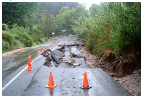
Washed out road from flooding
