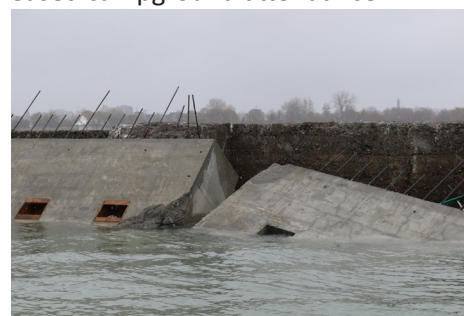
Buffalo, NY breakwall damage (USACE).
