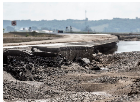
Iowa Highway 2 washed away in early June Missouri River flooding. (Iowa DOT)
