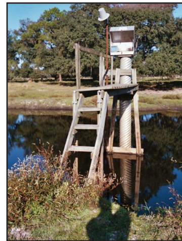
U.S. Geological Survey Stream Gage
