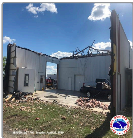
Damage from an EF-2 tornado in Franklin County, PA, on April 19. Image courtesy of National Weather Service State College.
