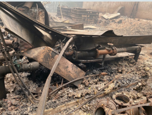
Sep. 2020 wildfire damage to a pump station at the City of Detroit, Oregon (top) and a water treatment plant facility at Panther Creek Water District, Oregon (bottom). Photo credit: Heath Cokeley, Oregon Association of Water Utilities Circuit Rider.
