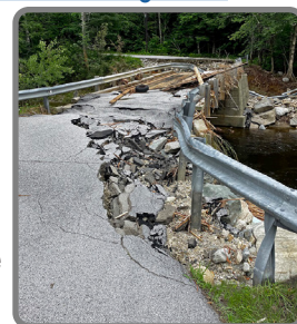
Flooding damage in Londonderry, VT. Credit: USGS New England Water Science Center .
