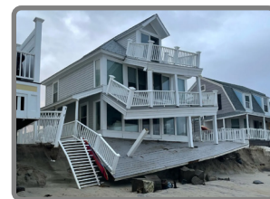
Damage in coastal Massachusetts in mid-January. Credit: Essex County Storm Report/MyCoast MA
