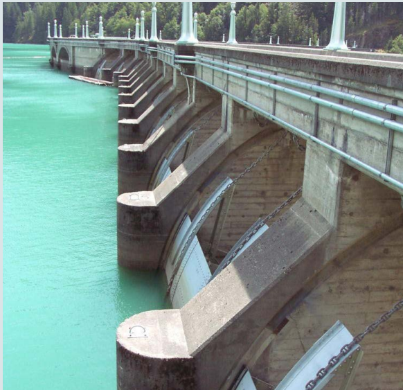
Diablo Dam, part of the Skagit River Hydroelectric Project in Washington. Credit: Dan Huntington, Creative Commons
